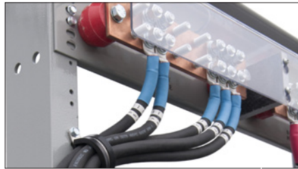
Cable harnesses and bus bar
